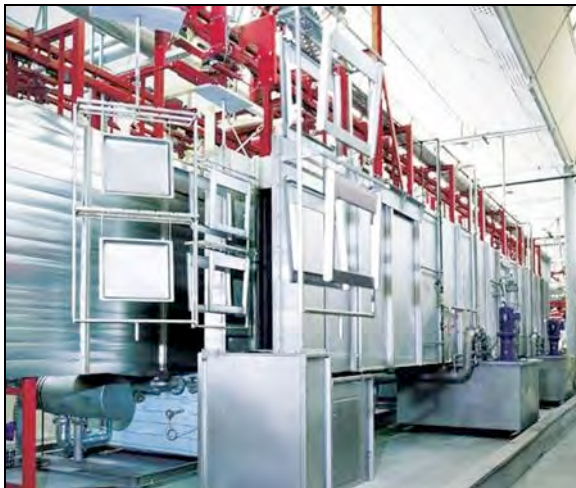
Figure 1 (Pretreatment / spray tunnel)
